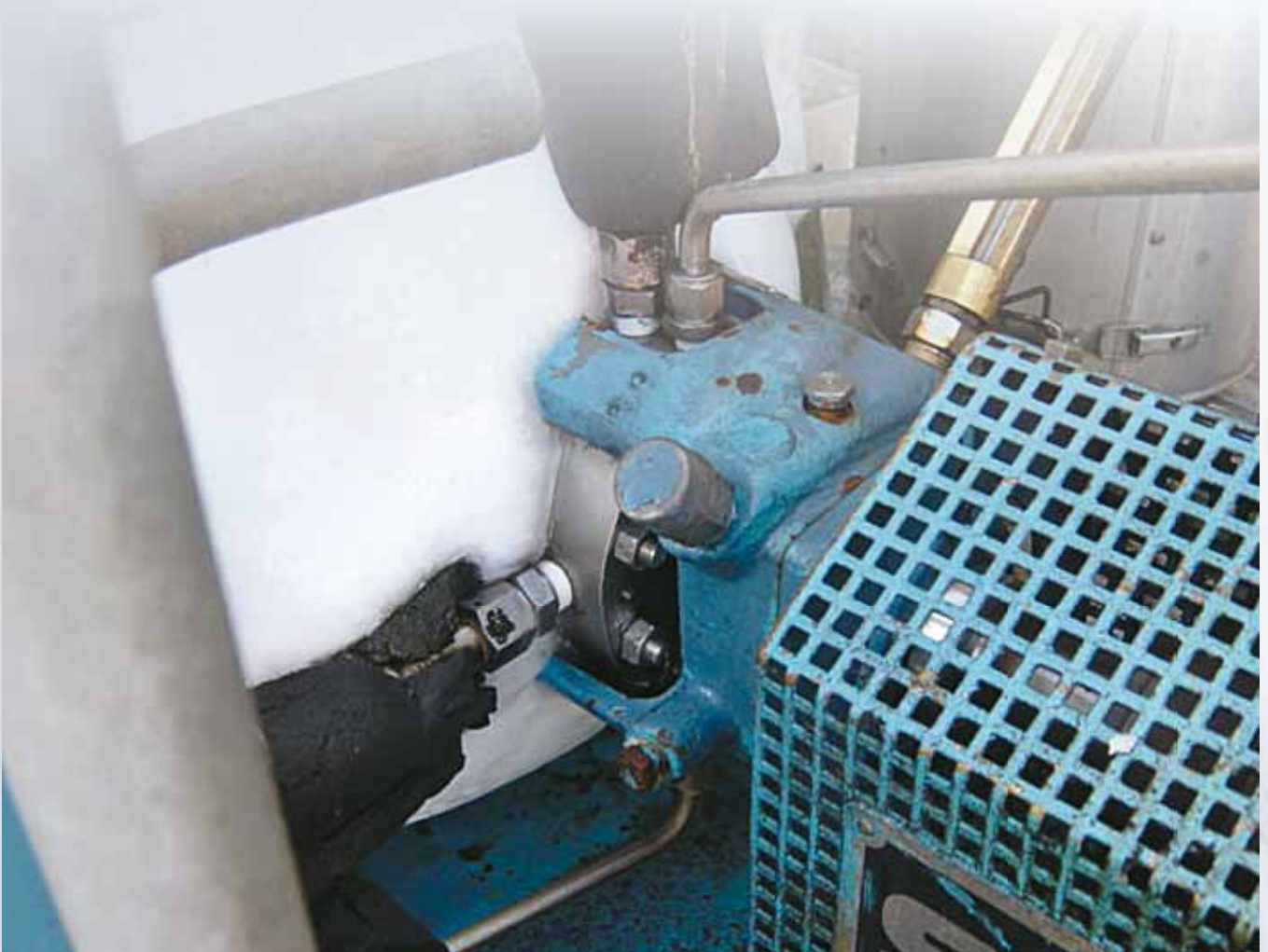
Ethylene pump with EagleBurgmann triple seal
